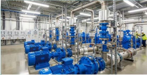
Chapter 3 Pumping Facilities
