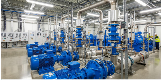
Chapter 3 Pumping Facilities
