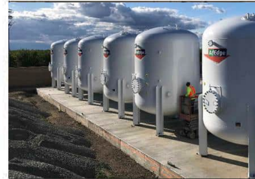
LARGE MODULAR TREATMENT SYSTEMS
