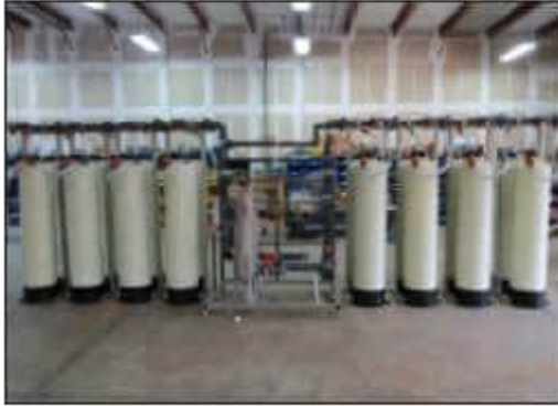
MODULAR TREATMENT SYSTEMS
