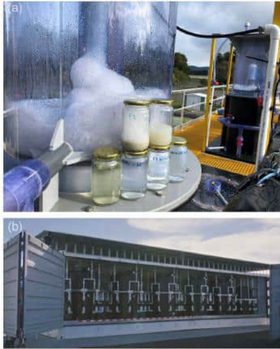
FIGURE 3 (a) Foam fractionation column treating PFAS-laden water (photo courtesy of Evocra Pty Ltd). (b) Foam fractionation system (photo courtesy of OPEC systems and Dora Chiang, CDM Smith)
