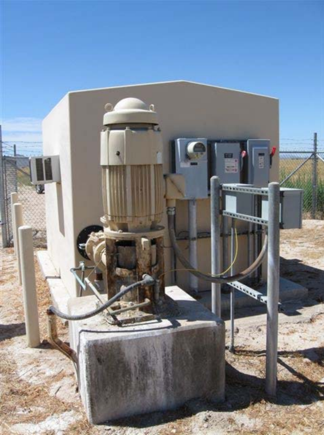
Extraction Well E-102
