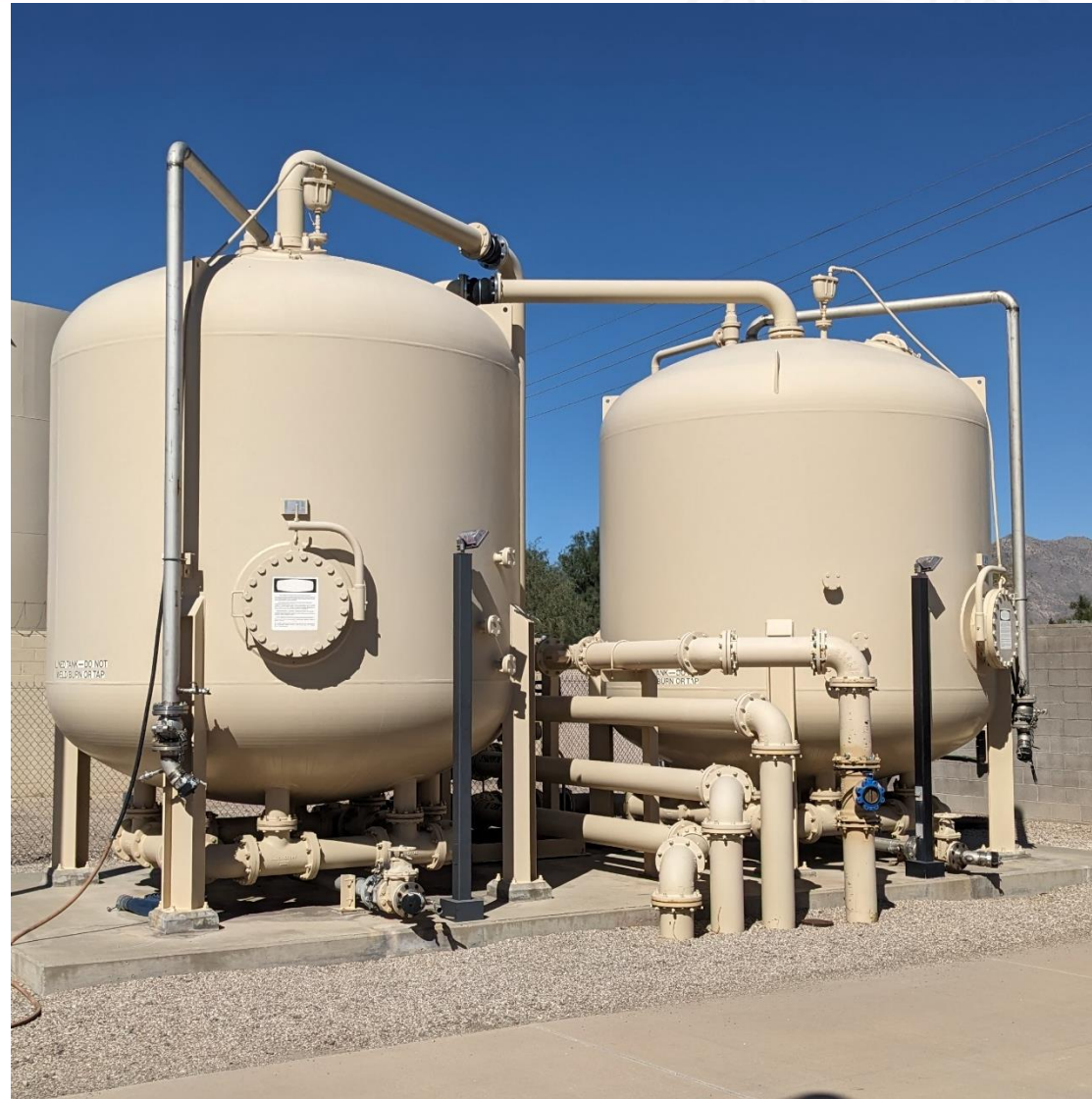
Existing carbon treatment vessels 10
