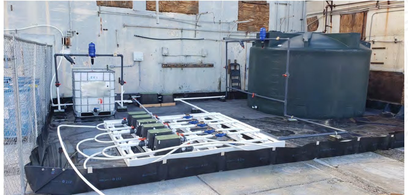
In-Situ Injection System at Lake Havasu & Holly WQARF Site
