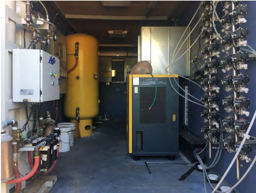
Ozone System at 24th & Grand Canal WQARF Site
