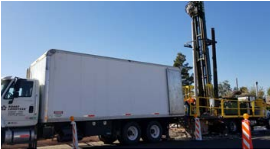
Installing groundwater monitoring wells at the 51st Avenue and Camelback Road WQARF Site.
