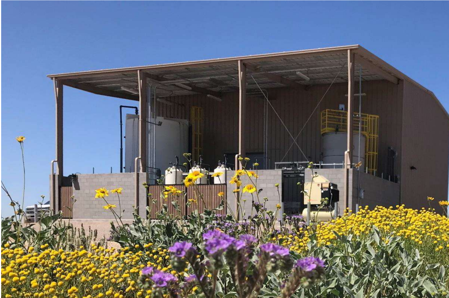
Figure 8- Groundwater Treatment Plant - Back
