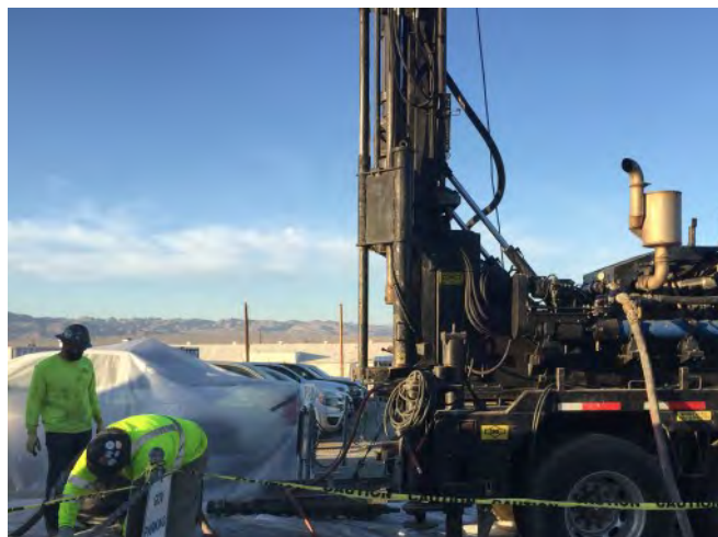
Routine maintenance is conducted on groundwater monitoring wells
