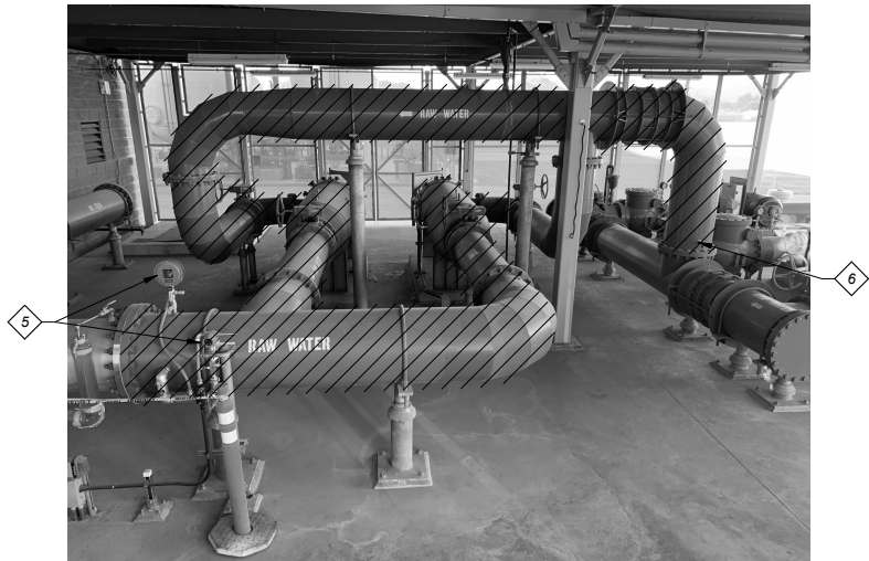
CARTRIDGE FILTER HOUSING & ASSOCIATED PIPING
