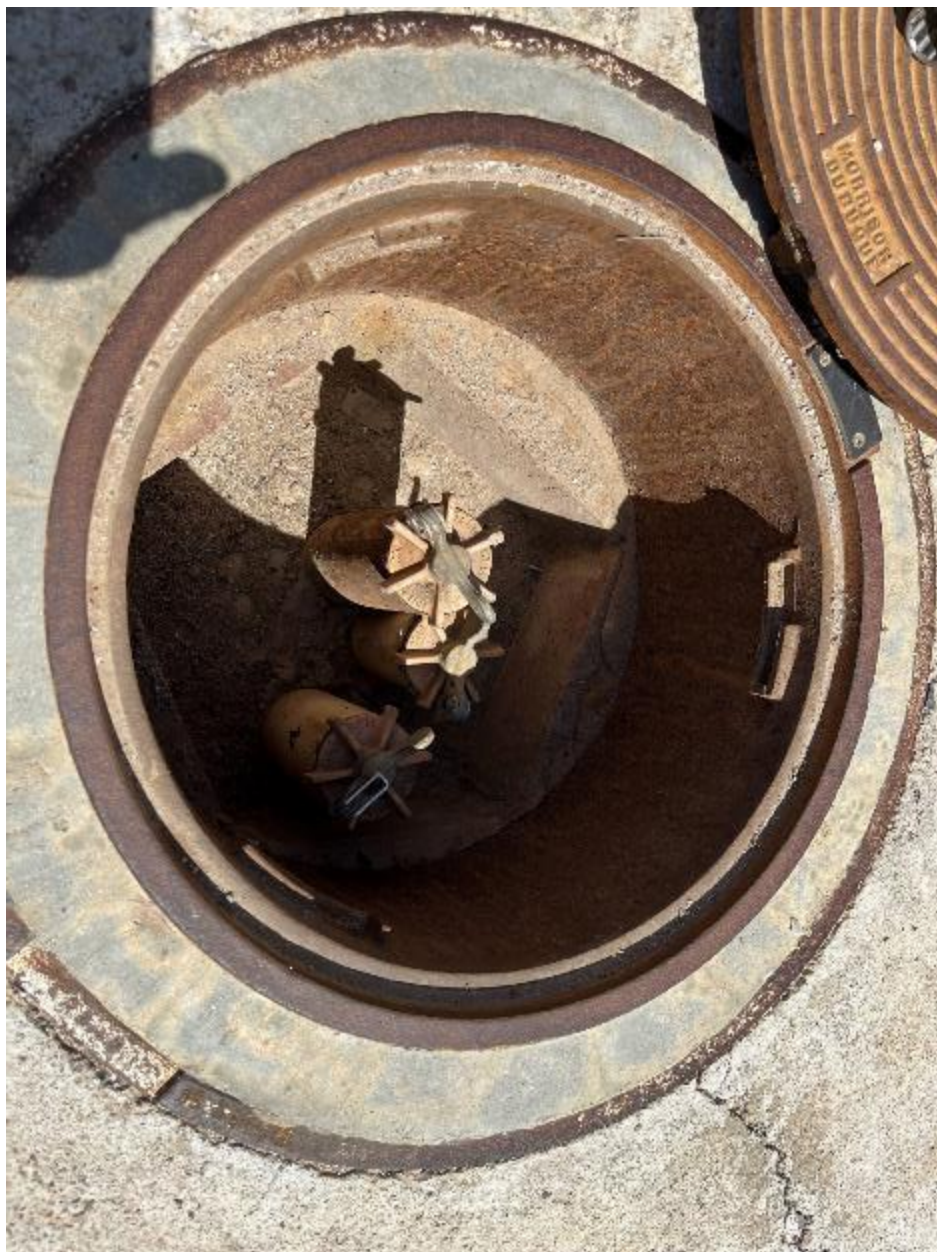
Figure 16- Airport Properties GWTP interior well vault CRA-3
