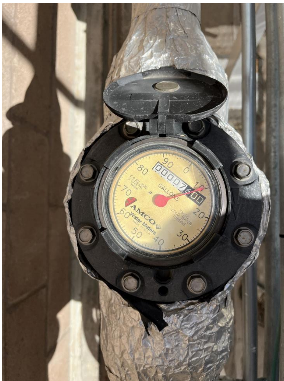
Figure 6- Airport Properties GWTP SVE totalizer
