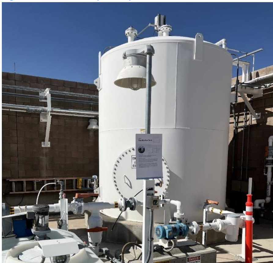
Figure 2- Airport Properties GWTP Equalization Tank
