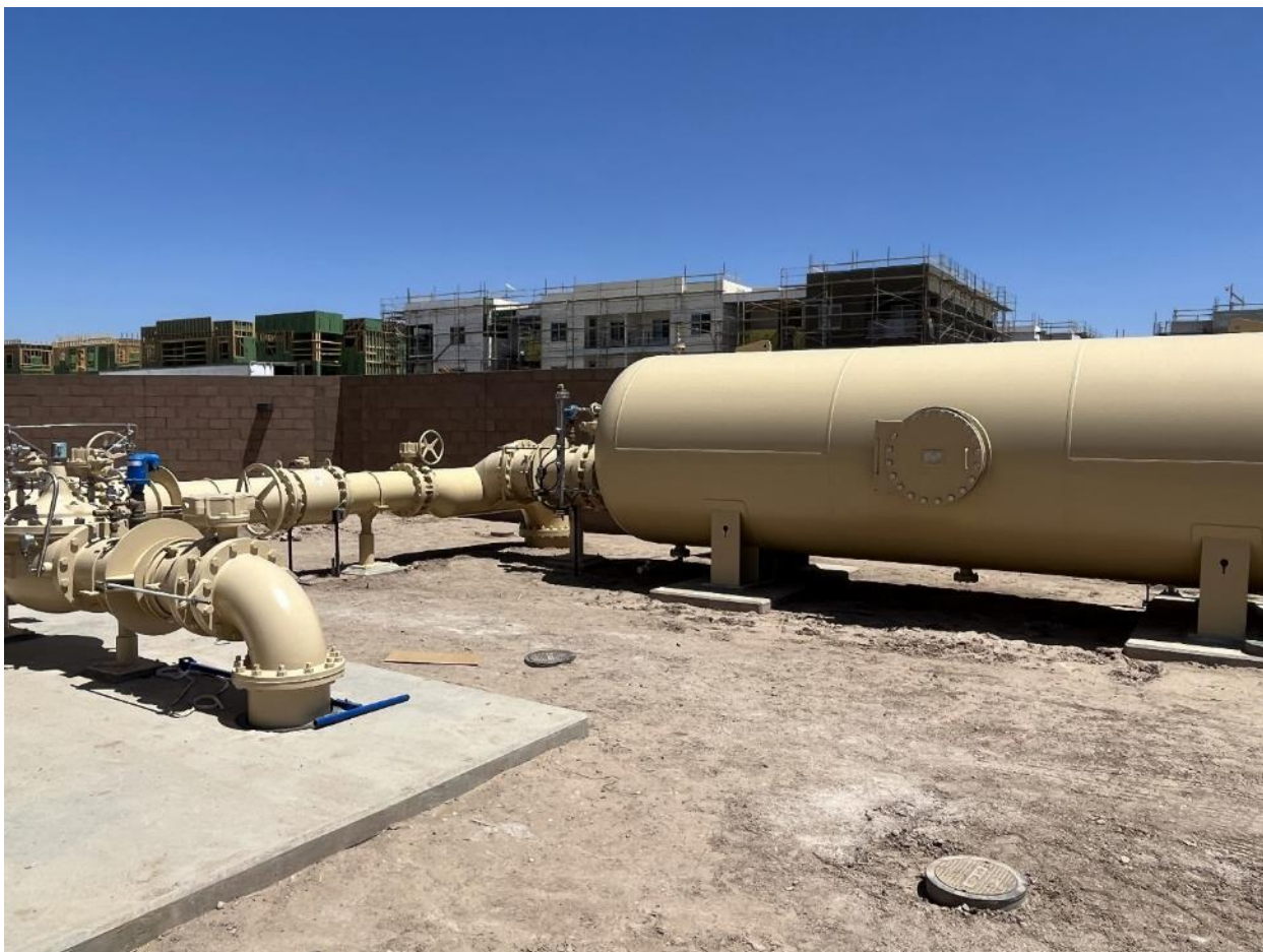
Figure 32- TARP connection to recycled water system.
