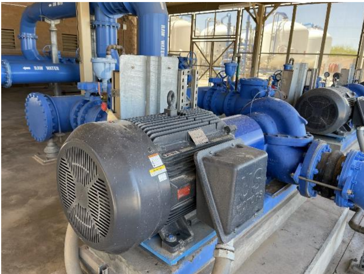
Figure 24- TARP system pumps
