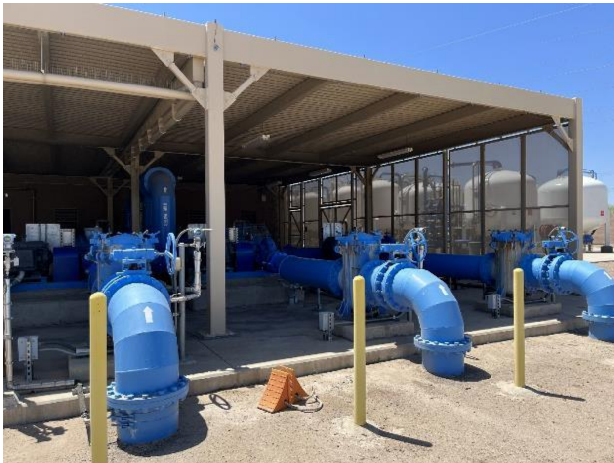
Figure 21- TARP inlet pipes
