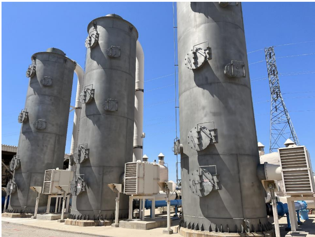
Figure 18- TARP PCA system (inactive)
