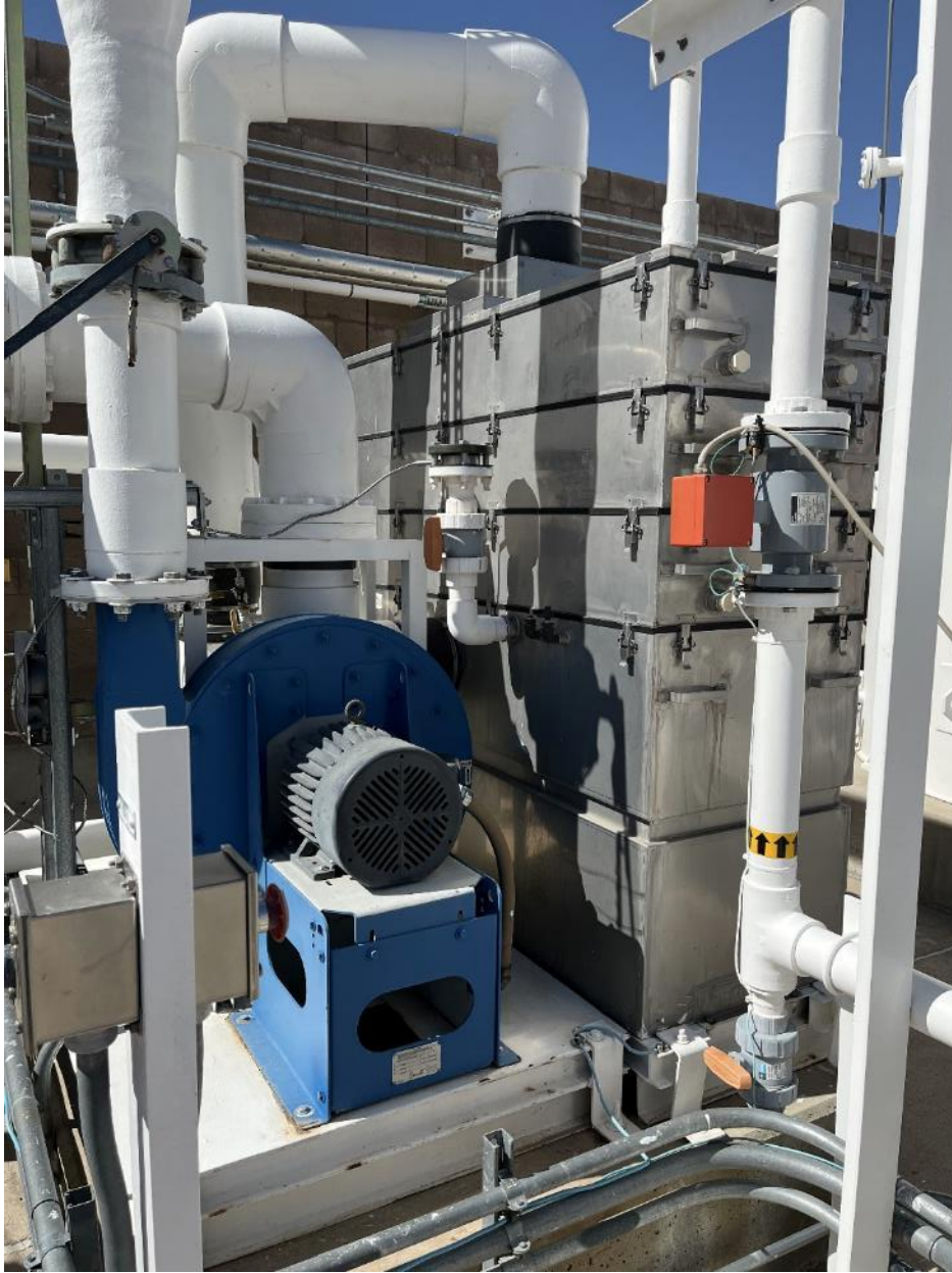
Figure 3- Airport Properties GWTP Air stripper
