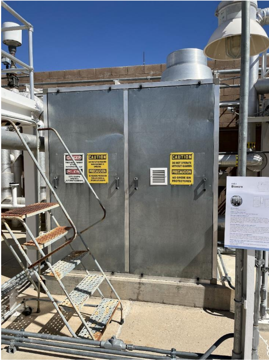
Figure 7- Airport Properties GWTP SVE blower cabinet
