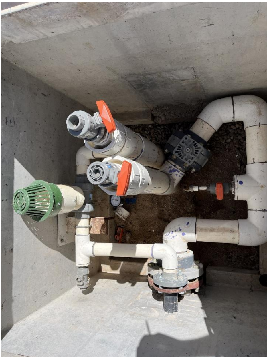
Figure 13- Airport Properties GWTP well vault SVE3
