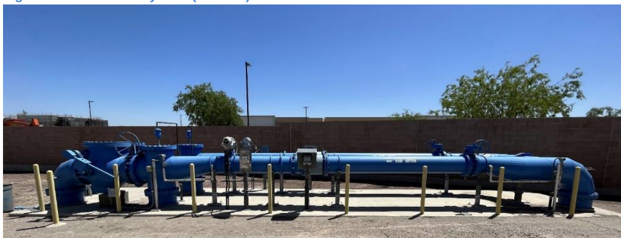
Figure 19- TARP influent pipe
