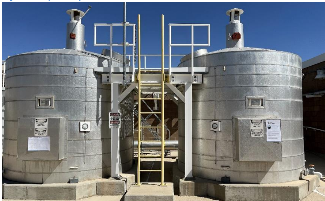
Figure 9- Airport Properties GWTP SVE carbon vessels
