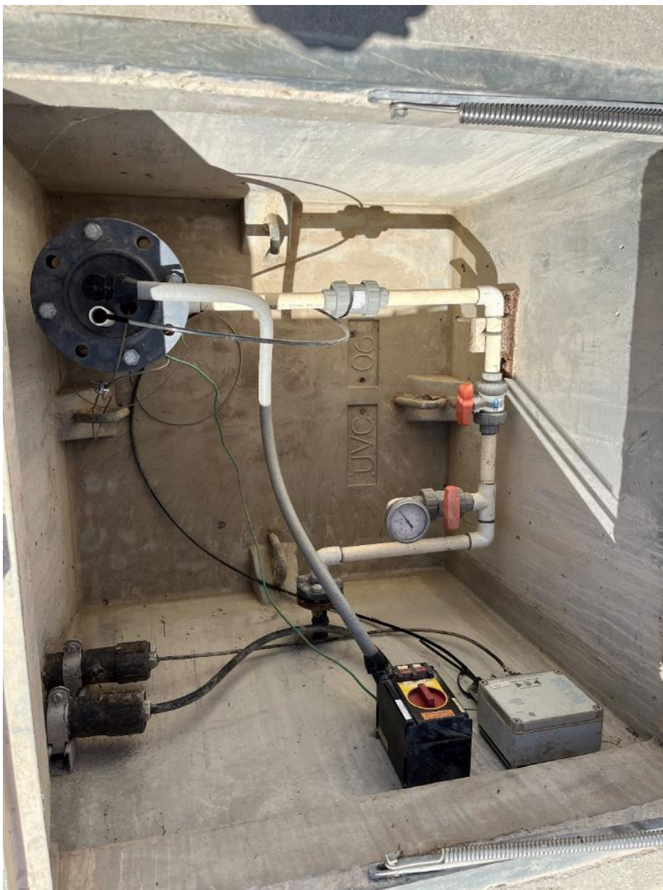
Figure 15- Airport Properties GWTP interior well vault CRA-5
