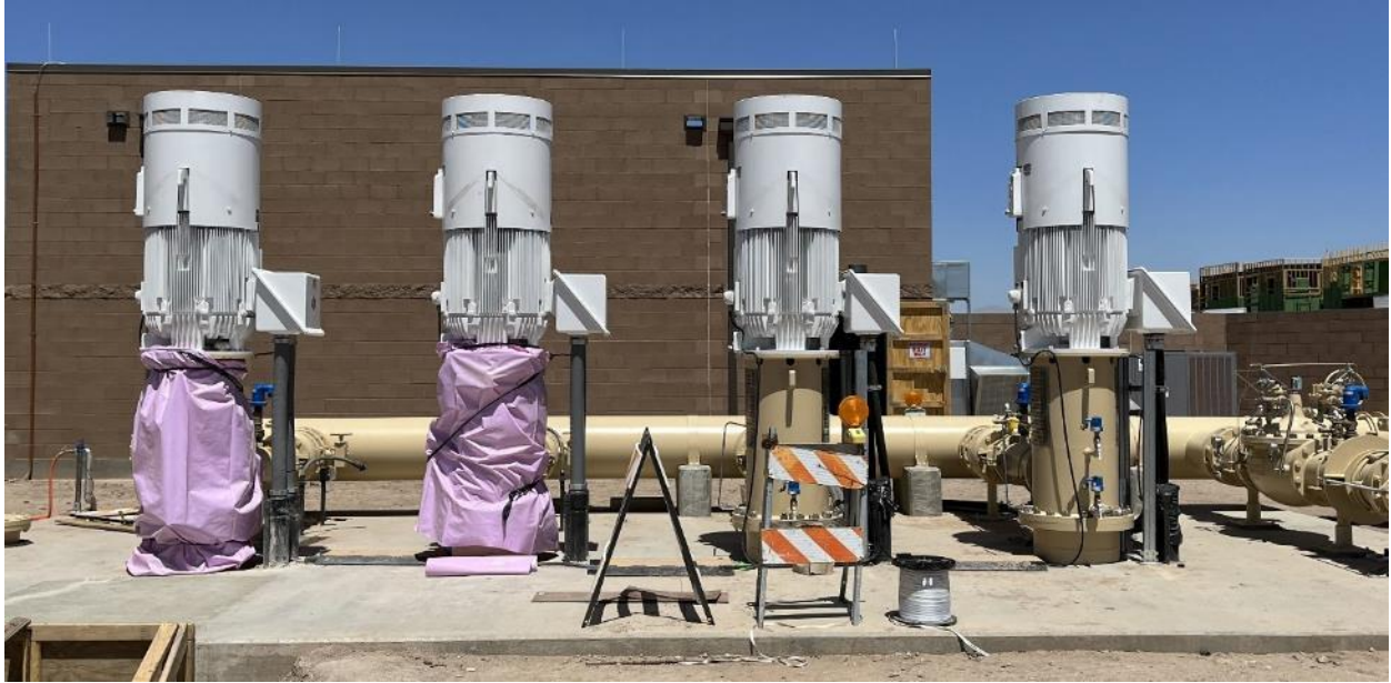
Figure 30- TARP effluent booster pumps
