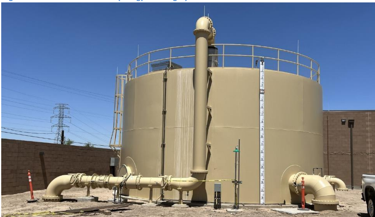
Figure 29- TARP effluent storage tank
