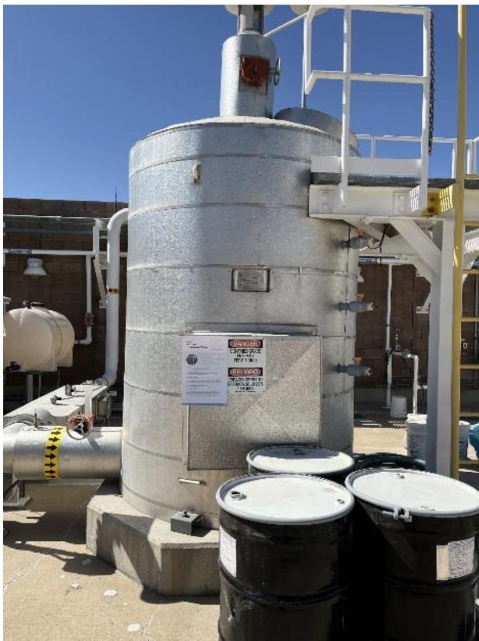
Figure 4- Airport Properties GWTP carbon treatment vessel
