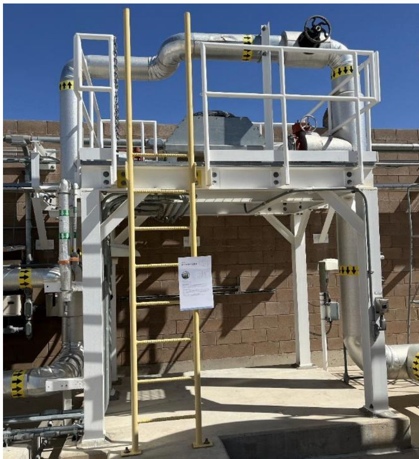
Figure 8- Airport Properties GWTP SVE air to air cooler
