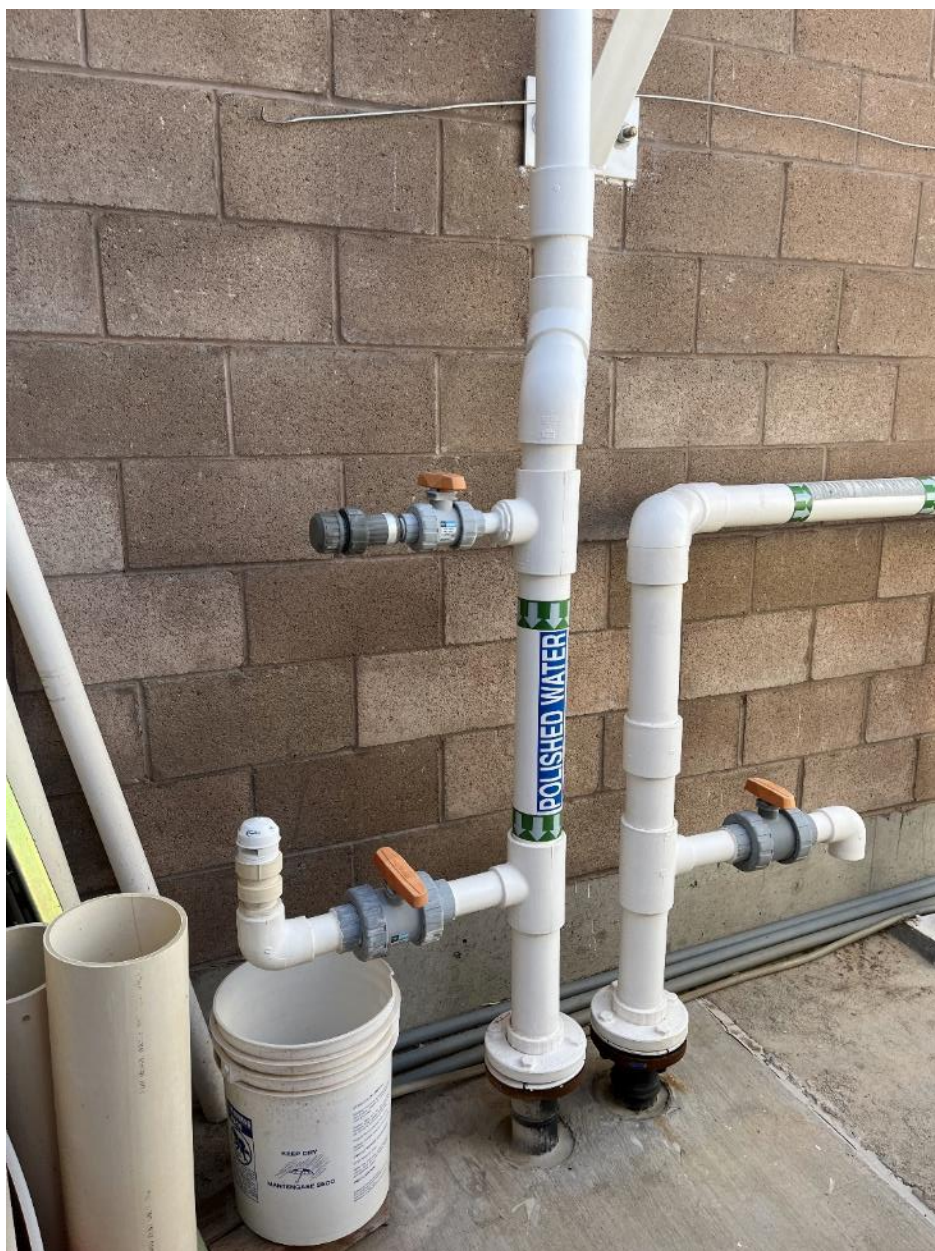
Figure 12- Airport Properties GWTP effluent line
