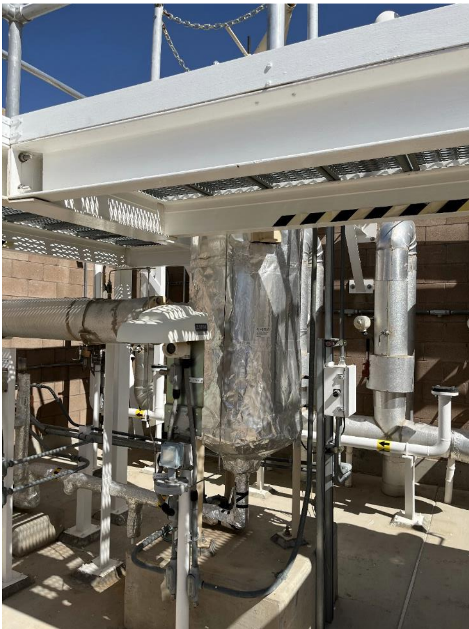
Figure 5- Airport Properties GWTP SVE knock-out pot.
