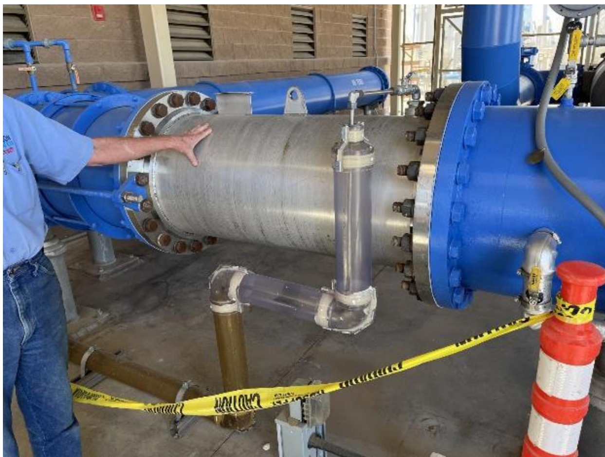
Figure 25- TARP peroxide injection point
