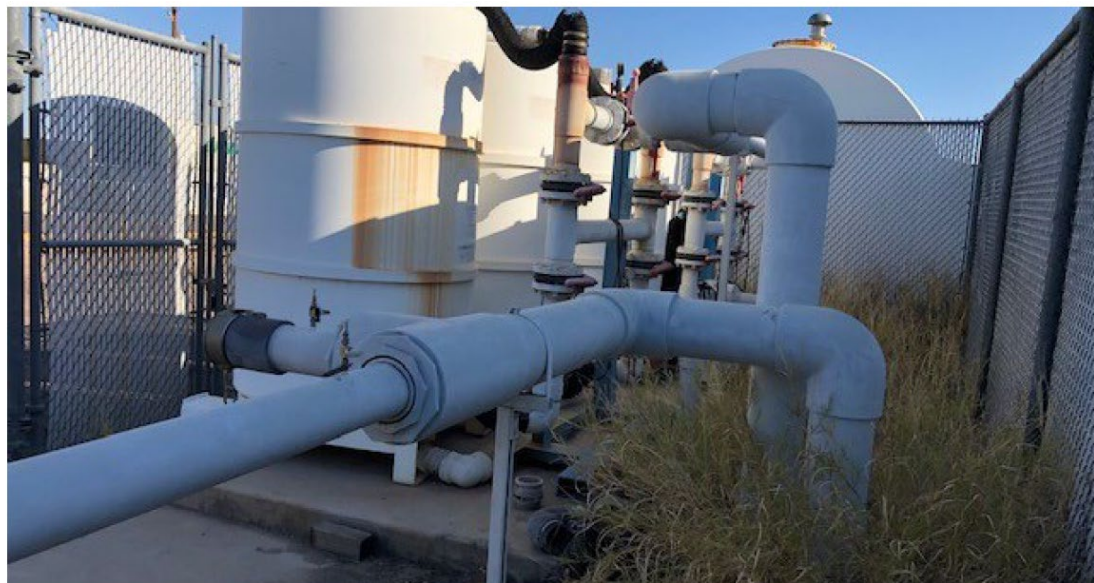
Photo 9 View of location of four carbon vessels and SVE piping before removal.
