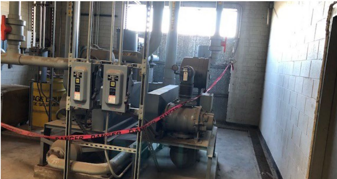
Photo 1 Soil Vapor Extraction (SVE) System in AD building.
