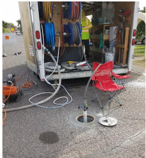
Typical trailer set-up for well injection
