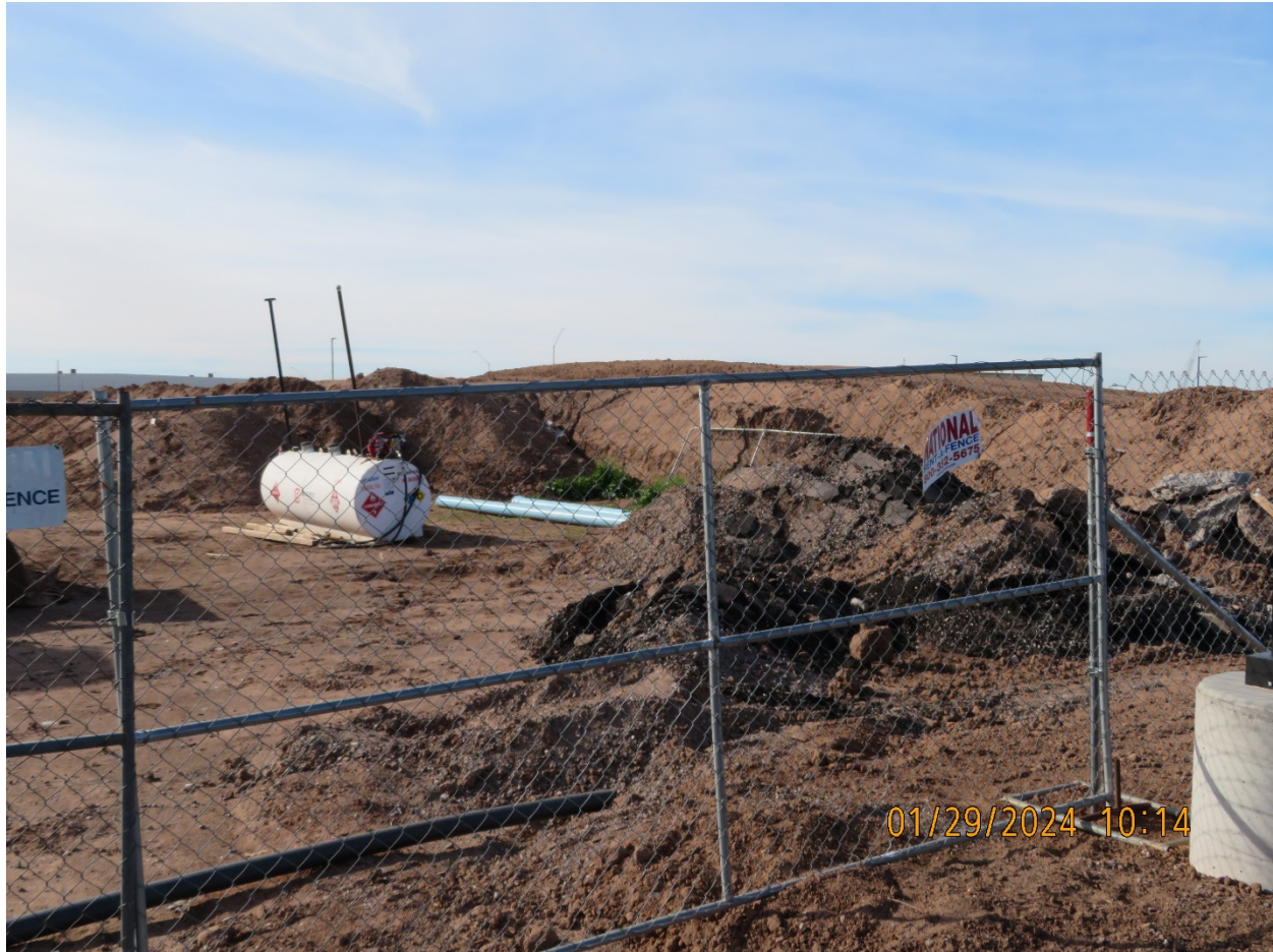
Photo 3 South-facing View of Dirt Lot with a Diesel Fuel Tank in Place for Construction Crew Working
