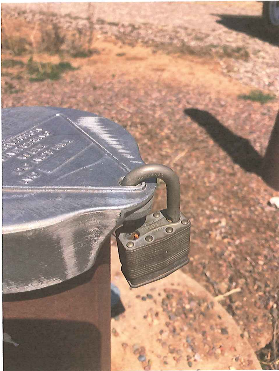
Picture 10 Unlocked SGD-DP wellhead
