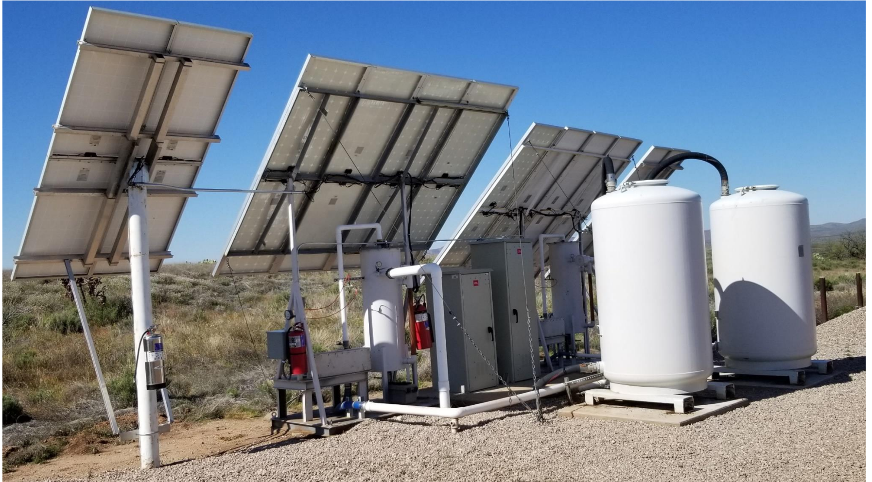
Figure 3: Picture of SVE System
