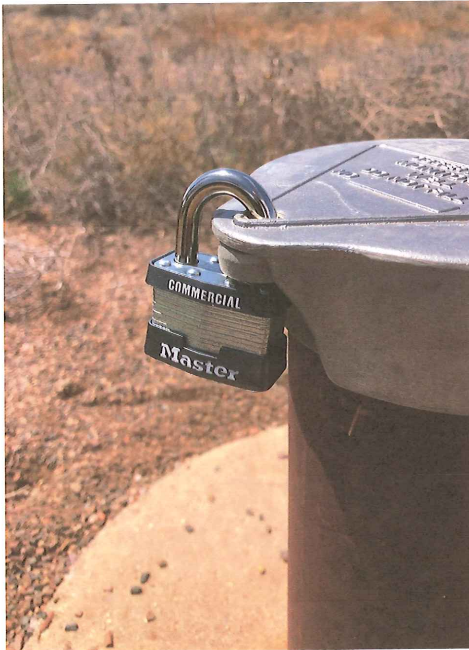
Picture 11 Locked SGD-DP wellhead
