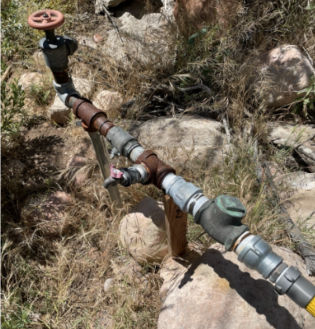
Figure 3. Hydrant overflow conveyance by hose.
