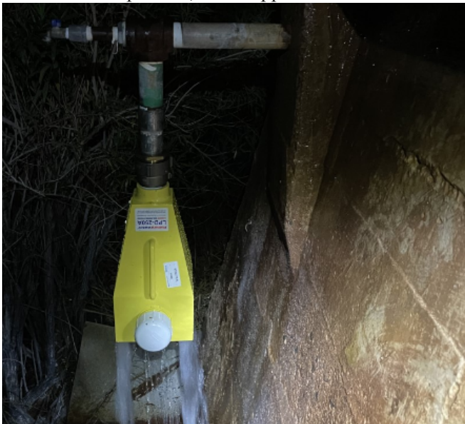
Figure 2. Discharge of effluent from Outfall 003 directly from LPD-250A dechlorinating diffuser, the final treatment process, at the upper Phantom Ranch area
