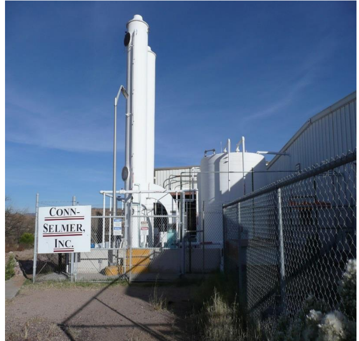
Figure 4 - Groundwater Remediation System (GRS); 1310 West Fairway Drive, Nogales, AZ. The GRS is fed by extraction well EW-2 (Figure 2) pumping at 50 to 75 gallons per minute (gpm) to an equalization tank with a containment capacity of approximately 7,000 gallons (right foreground). Water contaminated with low levels of volatile chlorinated organic solvents and degradation products (Table 1) is remediated via two air strippers, in series (left center). Remediated water is transferred to a 7,500-gallon retention tank for analysis prior to distribution to a lined surface impoundment managed by the City of Nogales. The GRS operates within an 8,150 gallon secondary containment, to capture any equipment spills. (ADEQ, 11/2008)
