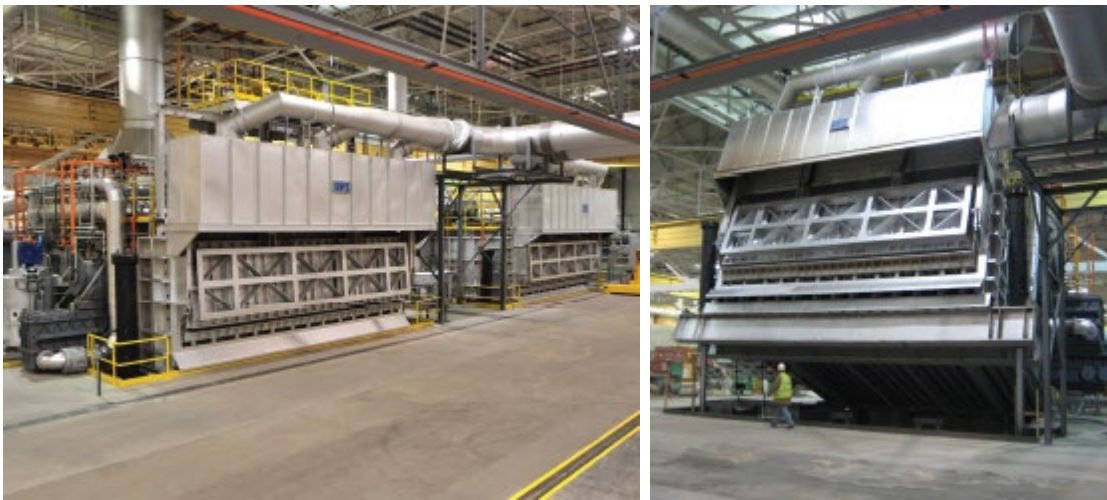
Figure 4-5. Pictures of Representative Tilting Holding Furnace
