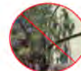
Tree branches touching storage tank
