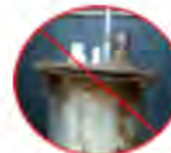
Well's sanitary seal in bad condition
