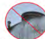
Hatch lacks a seal and a lock
