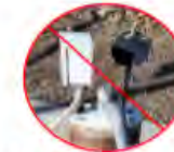
Missing raw water sample tap and air vent
