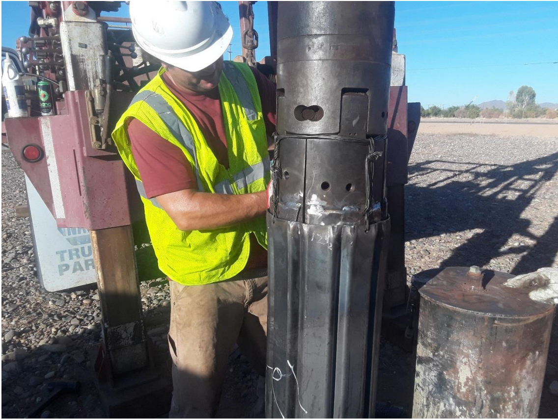
View of swage tool and bridge plug
