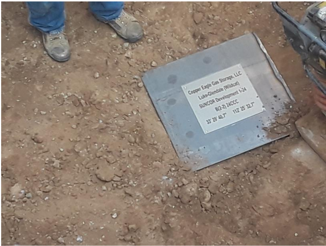
View of metal plate placed over tubular casing at base of 1-24 excavation
