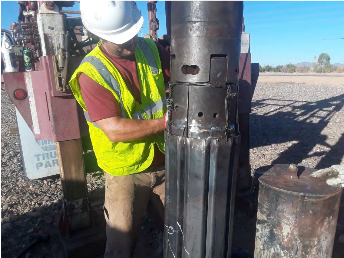
View of swage tool and bridge plug
