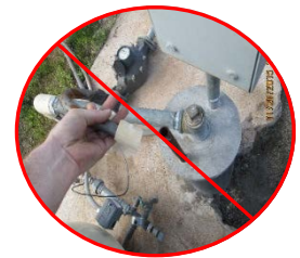
Broken air vent
