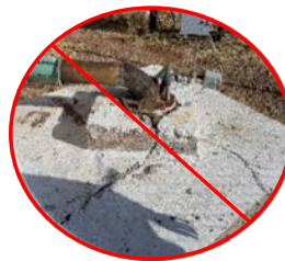
Cracked well slab
