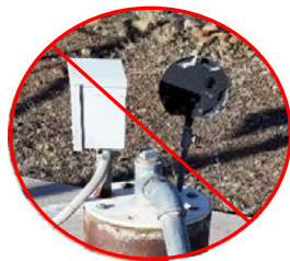
Missing raw water sample tap
