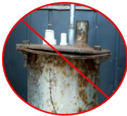
Well's sanitary seal in bad condition
