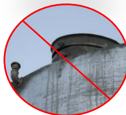
Hatch lacks a seal and a lock
