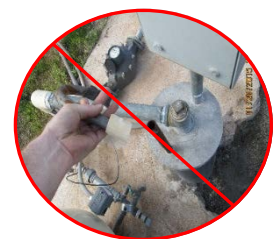
Broken air vent
