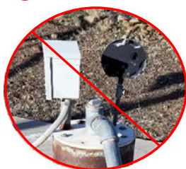
Missing raw water sample tap
