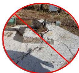
Cracked well slab
