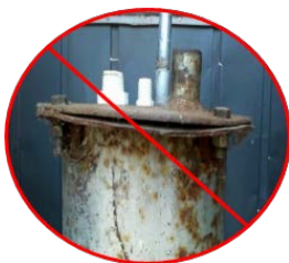
Well's sanitary seal in bad condition
