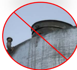
Hatch lacks a seal and a lock
