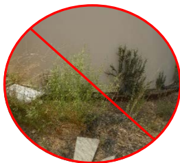
Excessive vegetation around storage tank
