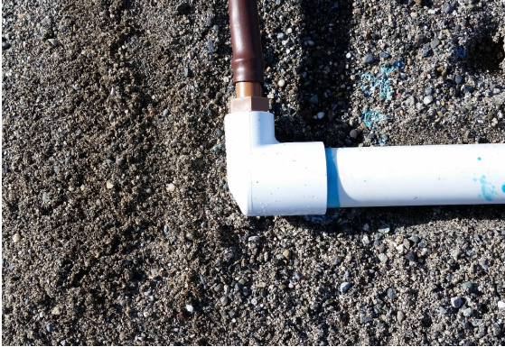
Manifold and blank tech line adapter and connection.
