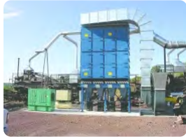
DLMC 4/8/15 Baghouse Dust Collector Rock Crushing
