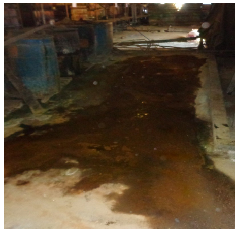
Leaks and spills can lead to hazardous constituents being tracked outside of the facility.
